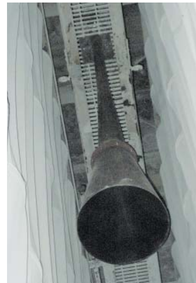
Bottom view of 60 Hz horns mounted under R/A baghouse walkway
