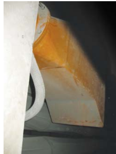
New 125 Hz sonic horns, mounted under Reverse Air (R/A) baghouse walkway
