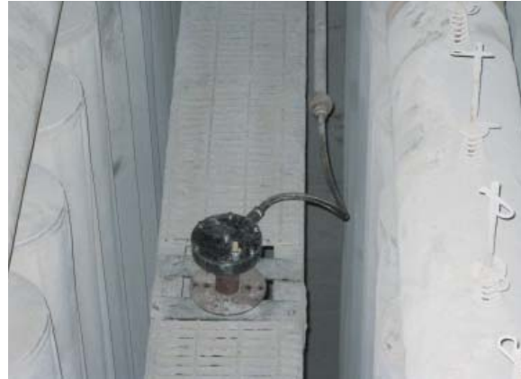
Top view of 60 Hz horns mounted under R/A baghouse walkway
