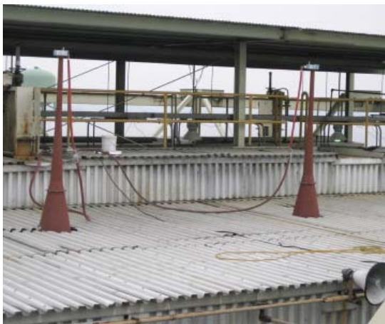
New roof-mounted 60 Hz sonic horns
